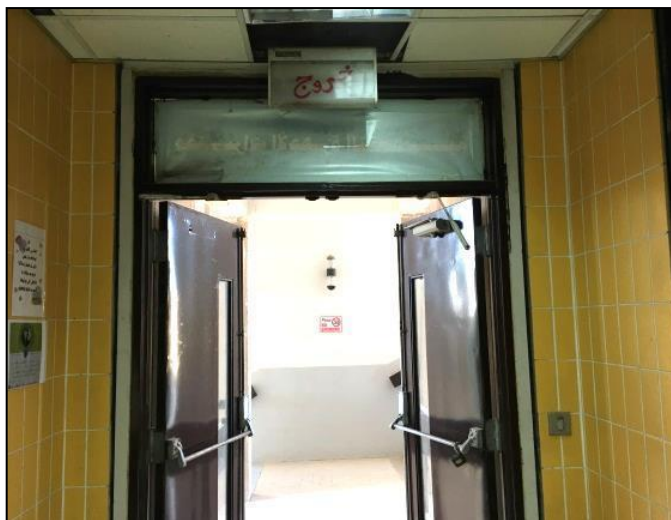
Figure 2: Opening the door of the emergency exit for evacuation.
